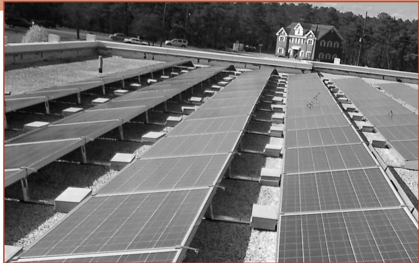
Solar panels installed on the roof of the Hooper Avenue Elementary School in the Toms River Regional School District provide an alternative energy source to power the building.
